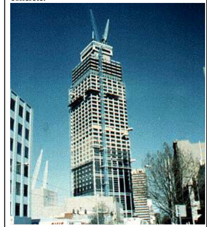
Figure 8 - Melbourne Central. Silica fume was used to provide high strength pumpable concrete.
